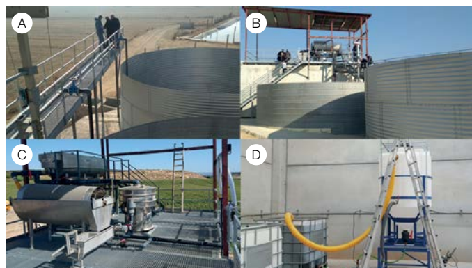
A, B and C: images of the SAT La Vall 100 m 3 pilot plant. D: 1 m 3 pre-pilot slurry treatment plant. Photos: Operational Group.
