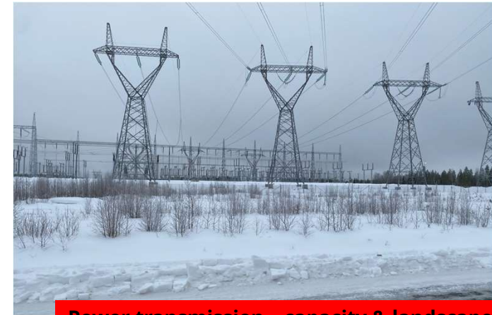
Power transmission – capacity & landscape?
