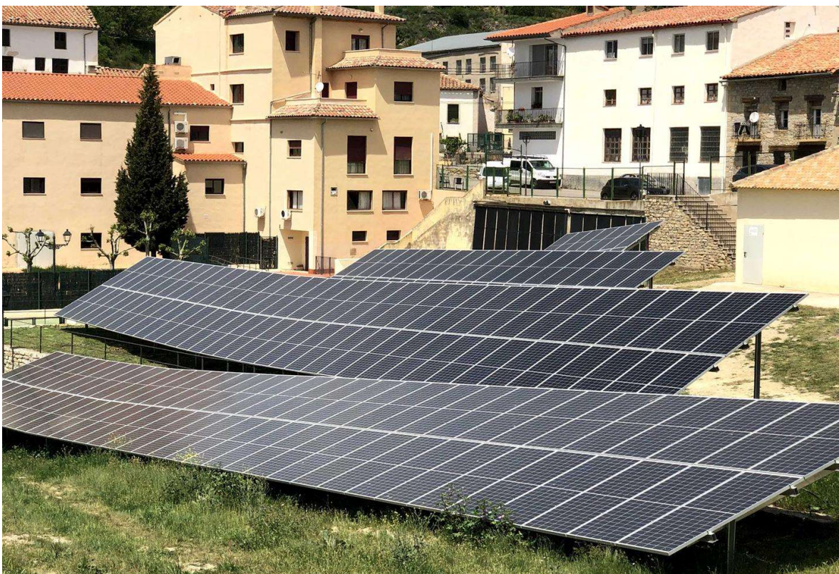
FV solar instalation in Portell de Morella
