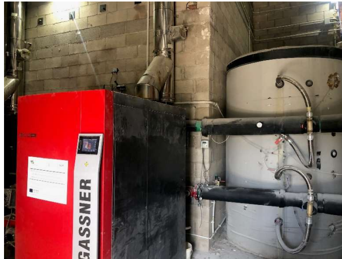
Boiler room and accumulation or buffer tank
