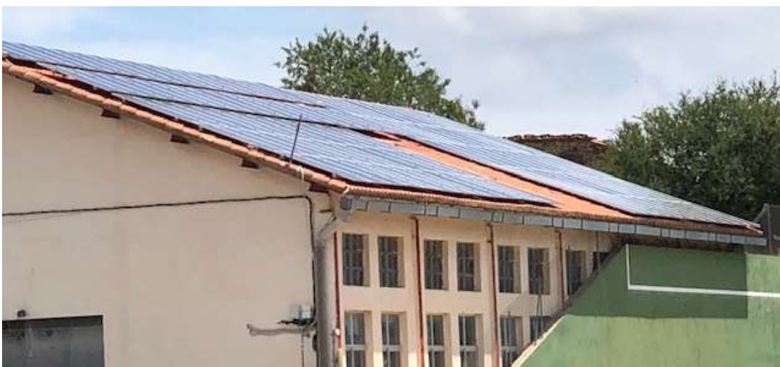
Self-consumption installation on the roof of the district-heating boiler building
