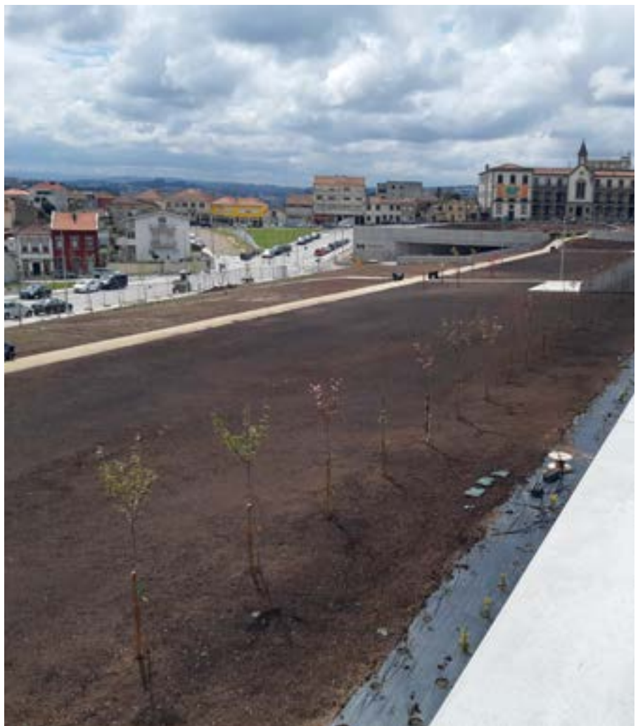
Campanhã Station Intermodal Terminal in Porto, Portugal (in construction) will also include extensive green areas. Picture: Janez Nared
