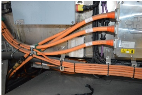
High voltage powerlines
