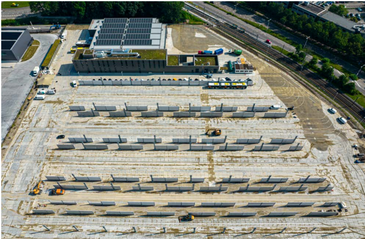
Concrete walls and a fire lane divide the charging compartments. Photo by Van der Ven, Brakel
