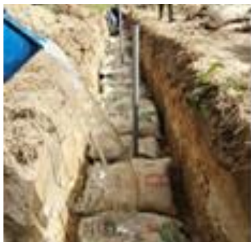
Figure 20 OMP vertical beds in the way of leachates running from a manure heap
