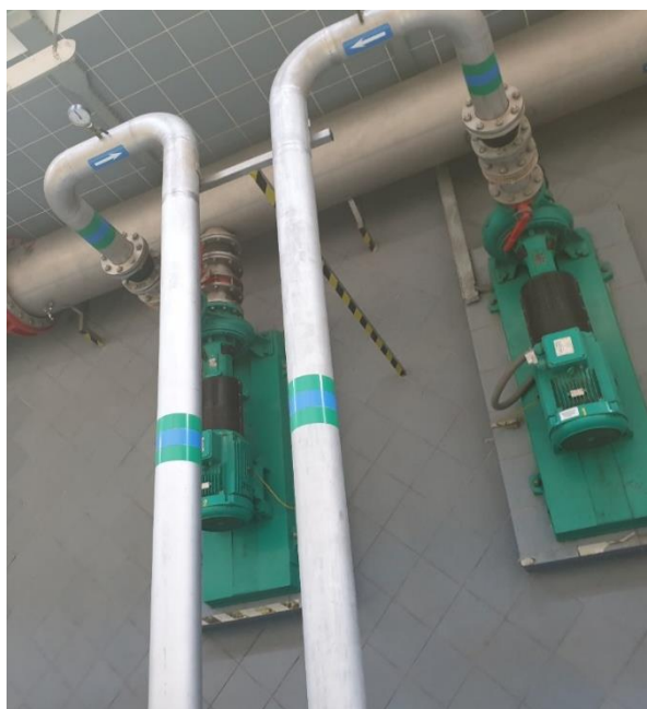
Figure 16 Clean water pumps feeding the water supply main of MPWiK Sieradz
