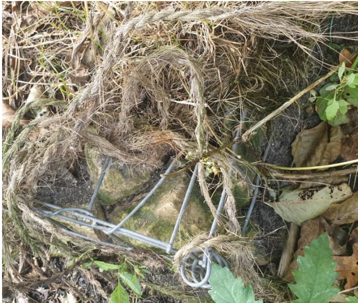
Figure 8 Geochemical filter: eliminates biogenic compounds by a geochemical structure (the underwater gabion zone filled with dolomite, limestone, and coconut fibre mats)
