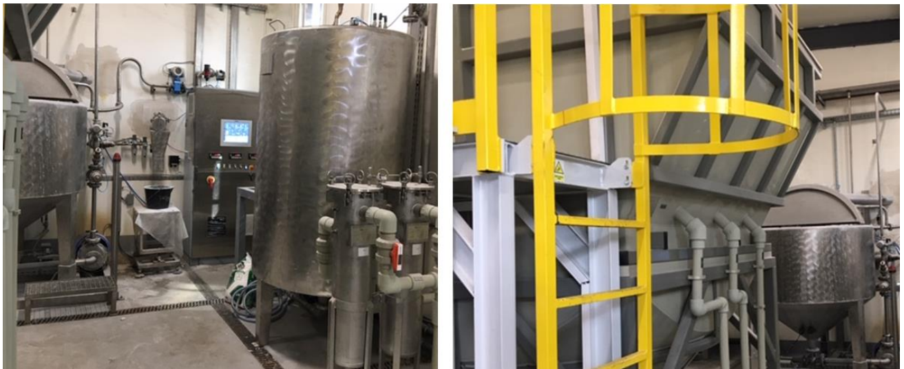
Figure 2 The BCSTP (biological and chemical sewage treatment plant) systems at Farbiarnia Bilińscy
