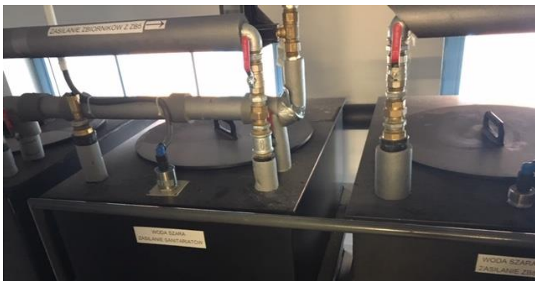
Figure 10 Water supply tanks at Level 4 of the EC1 Wess Switchgear Building
